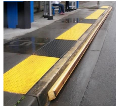
Figure 8: Rub Rail Swift BRT Seattle, Washington
